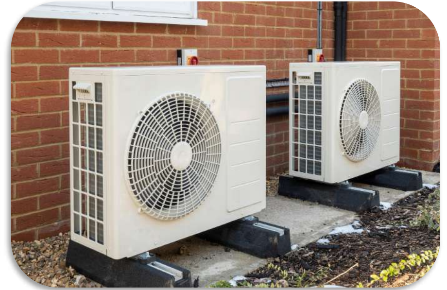
The outdoor unit of an Air-source heat pump
